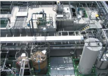
Wastewater treatment system
