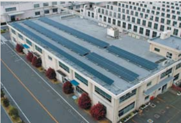
Photovoltaic power generating system at Yamaha's head office
